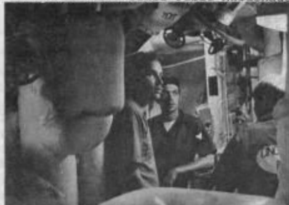
Framed by piping in the forward fire-room, Boiler Technician First Class Val Lipka and Boiler Technician Third Class Dan Schell listen as a Navy inspector from the Pacific Fleet Propulsion Examining Board explains his findings during LOE.
