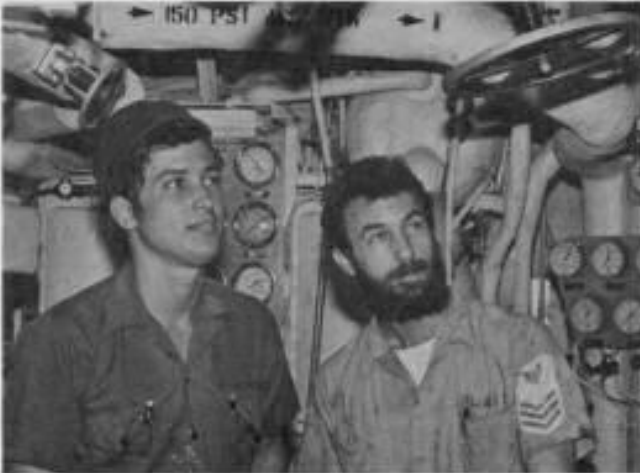
Surrounded by the multitude of gauges and controls in the after engine room, Machinist Mate Fireman Robin Henson and Machinist Mate First Class Paul Blain look pleased after the plant's successful performance during sea trials.
